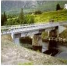
Bridges need to be stiff to minimize flexing under the application of applied loads
